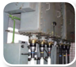
Power sensitive equipment
